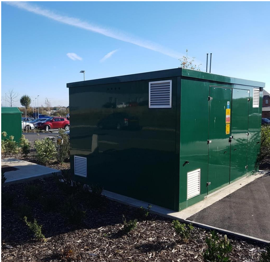
Figure 38 – An example of how a large above ground installation should be finished
