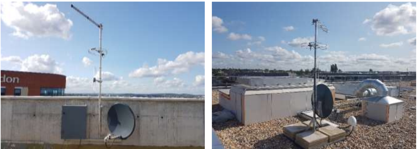
Figure 10 – Typical roof top deployments
