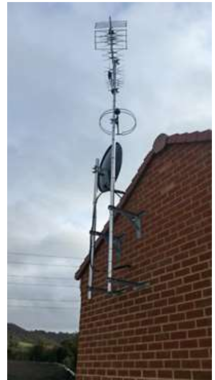
Figure 9 – A typical satellite dish, DVB-T and DAB antenna installation on an OSCP/substation building
